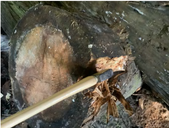
Tiebacks - typical rot
